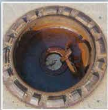
Water overflow causes cap release & leakage into tank
